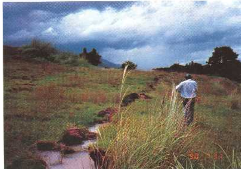
Fig. 4 13 - Ground ruptures damaging the Dalton Pass road at km 173+150 (top), km 178+000 (center) and near km 180 (bottom). Courtesy of DPWH and Katahira.
