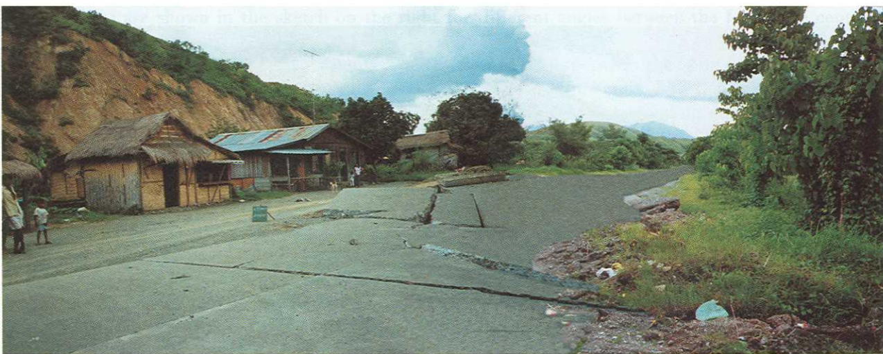
Fig. 4.14 – Faulting in Digdig, at the junction for Carranglan village (km 181+950 of the Maharlika Highway), with 4.8 m horizontal and 1.5 m vertical displacements (top). Fault crossing the road at km 182+700 (center) and at km 183+200 (bottom). Courtesy of DPWH and Katahira.
