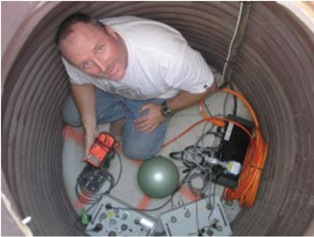
Figure A1.2. IDA field engineer installs the NGS equipment in a vault in Saudi Arabia (RAYN).
