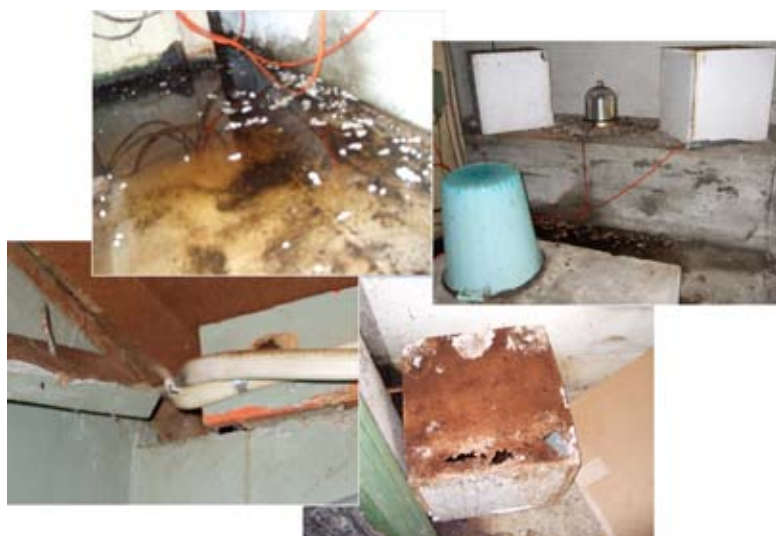
Figure A1.5. GSN station AFI (Afiamalu, Samoa) vault infrastructure issues (courtesy of ASL/USGS).
