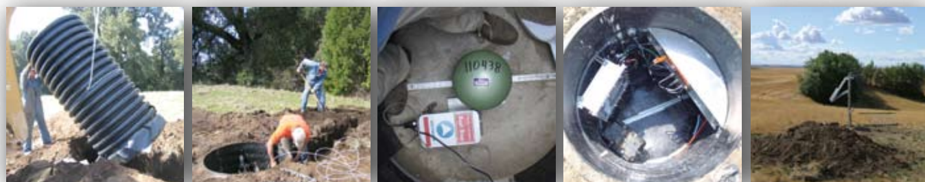
Figure A5.2. Installation of a Transportable Array station (left panels), instrumentation (middle and middle right panels), and completed station (right panel). The vault is under the mound of dirt in the foreground.
