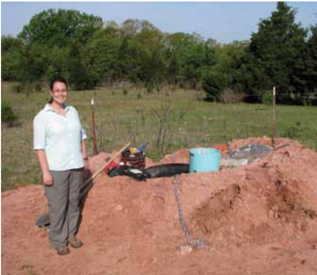
Figure 1: Catherine Cox at a TA station installation.
