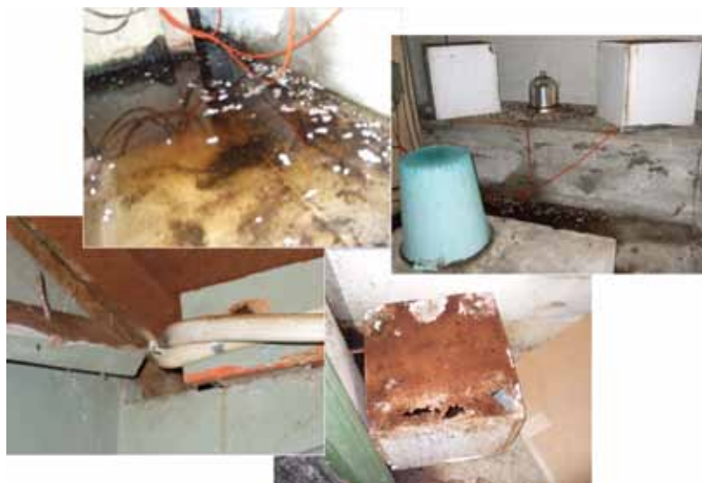
Figure A1.5. GSN station AFI (Afiamalu, Samoa) vault infrastructure issues (courtesy of ASL/USGS).
