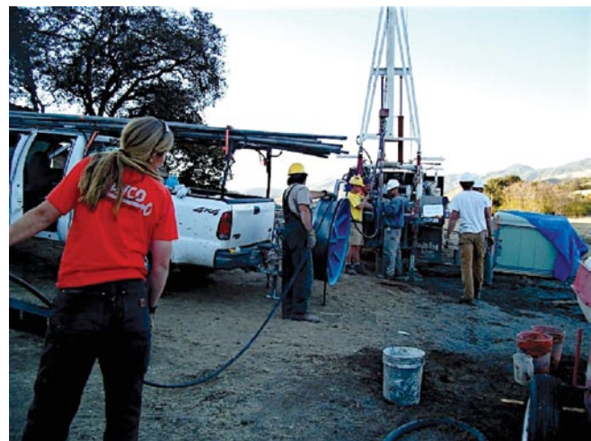
Figure 1.7. A PBO borehole strainmeter/seismometer installation along the San Andreas Fault near Parkfield, California. Engineer in the foreground is spooling out strainmeter cable as the instrument is being lowered into the borehole using the derrick lift in the background.
