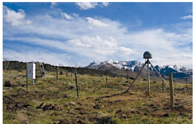
Figure 1.5. Completed GPS station near Delta Utah and the Wasatch Fault Zone. DDBM with radome housing GPS antenna is on the right. Enclosure housing GPS receiver and cellular modem is on the left. Security fence prevents equipment damage by livestock.
