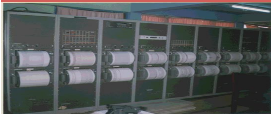
Central Recording Station at GGS HeadQuarters, Accra
